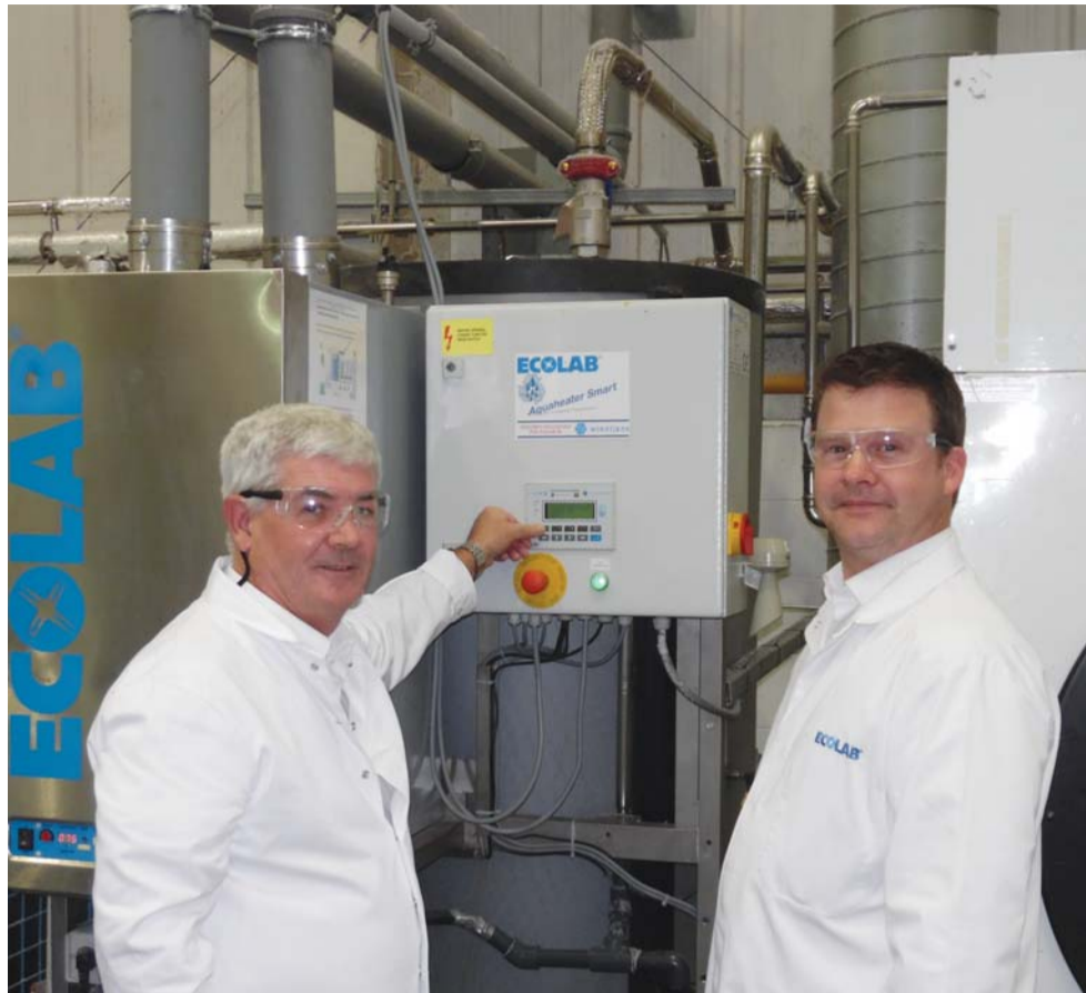
Pat O'Donnell (L) with Lee Shortland at the control panel of the Ecolab Aquaheater Smart which heats with minimum energy cost the water for the five washer/extractors in the Fishers Plant
