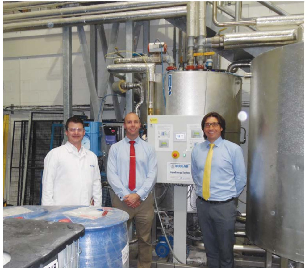
(L to R) Lee Shortland, (Ecolab), John Welford, Fishers Tyneside plant manager, and Mark Ferguson, operations manager, Fishers Tyneside Plant, in front of storage water tanks with pre-heated hot water stored for the batch washers
