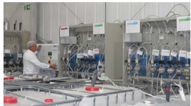
Pat O'Donnell, Ecolab technical support, checks settings on some of the dosing pumps for the OxyGuard40™ at Fishers Tyneside plant
