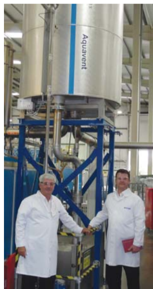
Pat O'Donnell(L) and Lee Shortland (Ecolab technical support staff) dwarfed by the imposing height of the Ecolab Aquavent System, which utilises the waste heat energy exhaust from the ironer lines to heat water for the batch washers – with massive cost saving to the laundry
